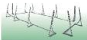
1 Assembly of the legs and the lower parts of the metal frame
